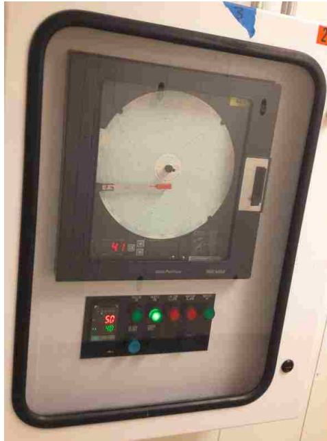
Figure 3.4.6.1 Control system of the freezer room
